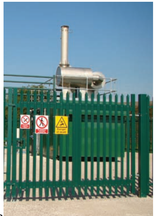
Generator at Doe Green >
