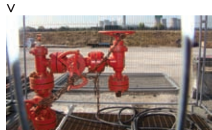
Well head at DG1
